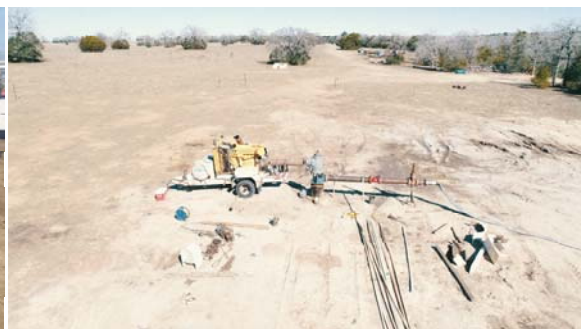
Well No. 8 36-Hour Pump Test
