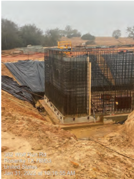
WTP/RWI – Recycle Pump Station
