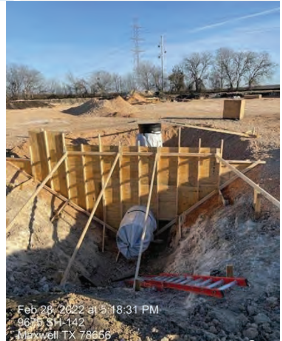
Outlet piping at GST
