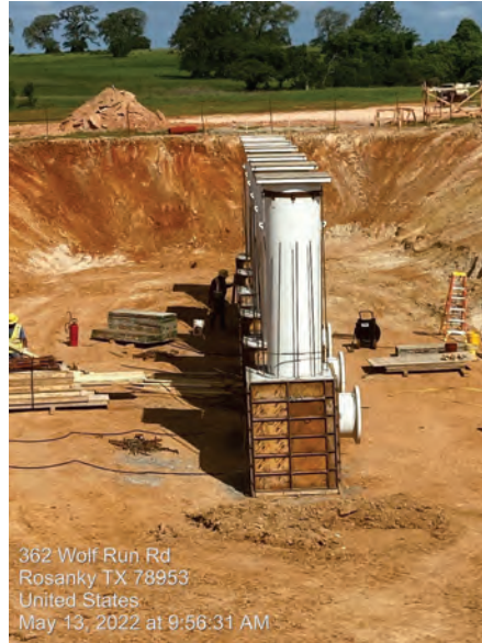
WTP– HSPS Pump Can encasement
