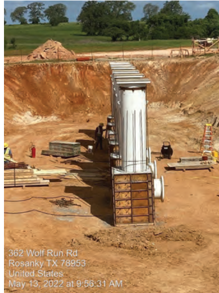
WTP– HSPS Pump Can encasement
