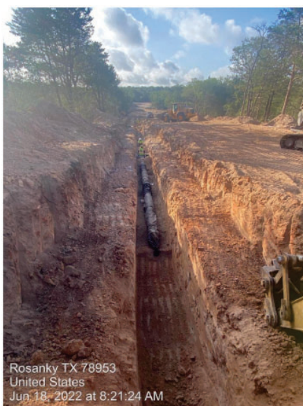
WTP – Raw Waterline WL-C
