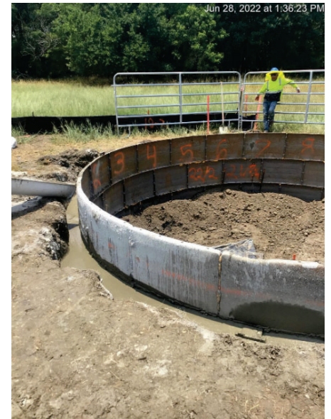
Seg A – Plum Creek Receiving Pit
