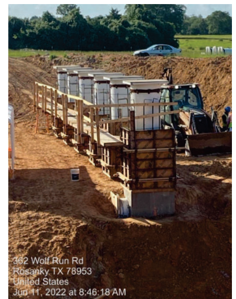
WTP – High Service Pump Cans
