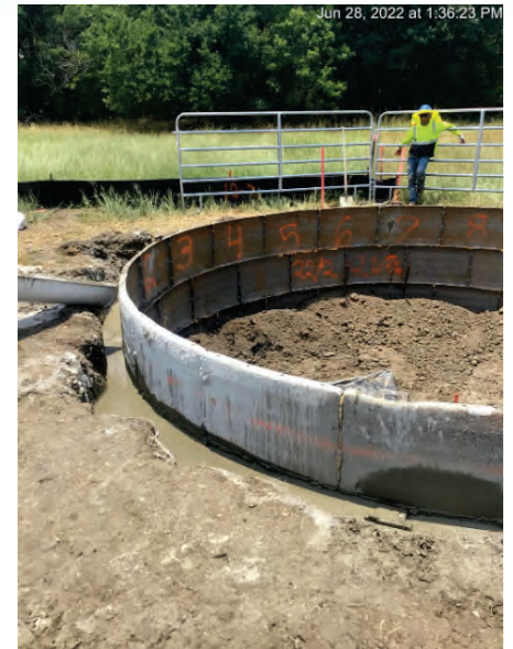
Seg A – Plum Creek Receiving Pit
