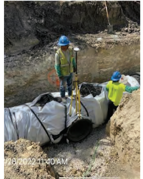
BPS – Segment B1 42" DIP at STA 12+71
