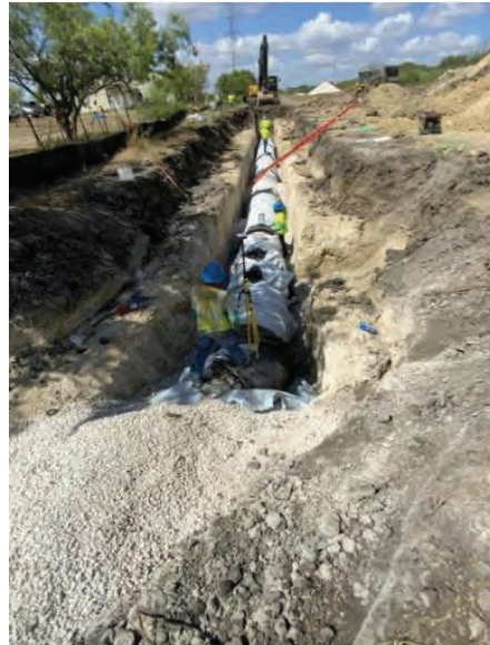
BPS – Segment B1 42" DIP at STA 11+67
