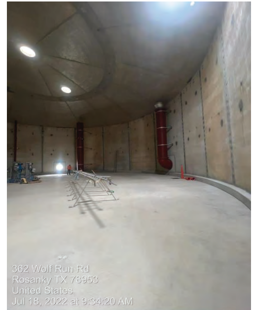
Raw Water Tank Interior Inlet and Overflow Piping
