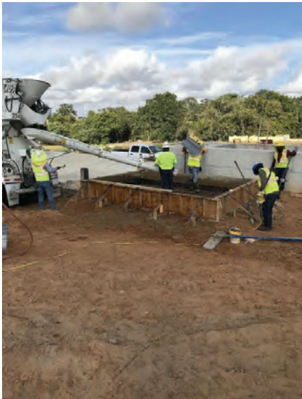
WTP – Plate Settler Basin Sludge Pump Pad
