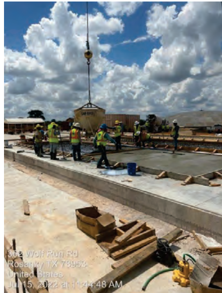
WTP– Filter Unit Housekeeping Pad of Filter Complex
