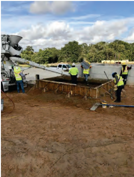
WTP – Plate Settler Basin Sludge Pump Pad
