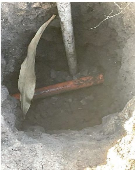
Seg B – Fiber Optic Line at Vista Ridge
