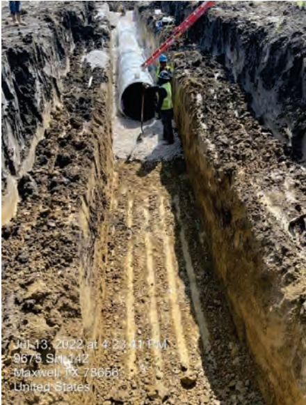
Segment B 36" DIP at STA 11+60
