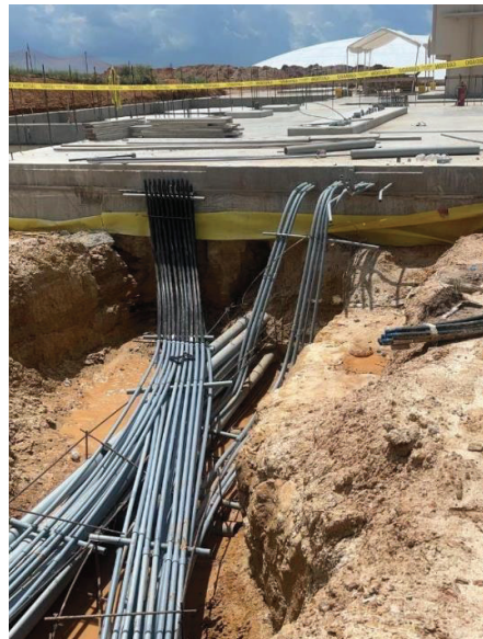
WTP – Electrical Conduits Entering Filter Complex
