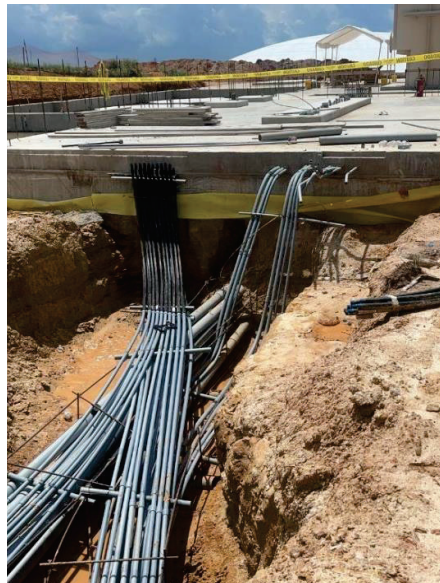
WTP – Electrical Conduits Entering Filter Complex
