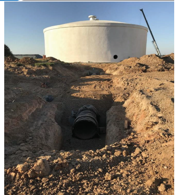
WTP - 36" GW Line to Raw Water Tanks
