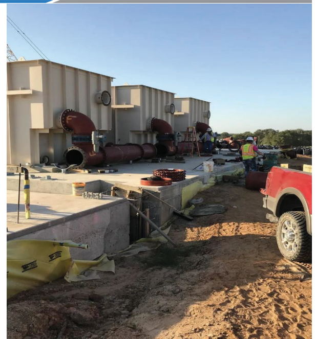
WTP - Filter Unit Process Piping
