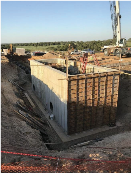
WTP – Rapid Mix Basin
