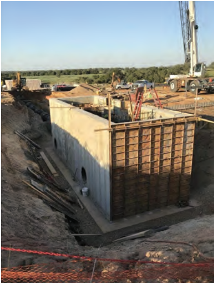
WTP – Rapid Mix Basin
