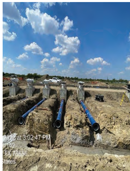
BPS – Pump Station Suction Piping to Pump Cans
