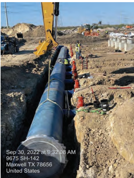
BPS – Pump Station Suction Header
