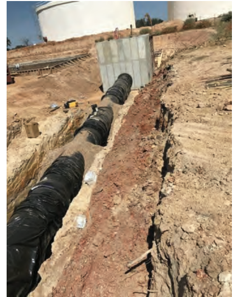
WTP – 42" Influent Line from Rapid Mix Basin
