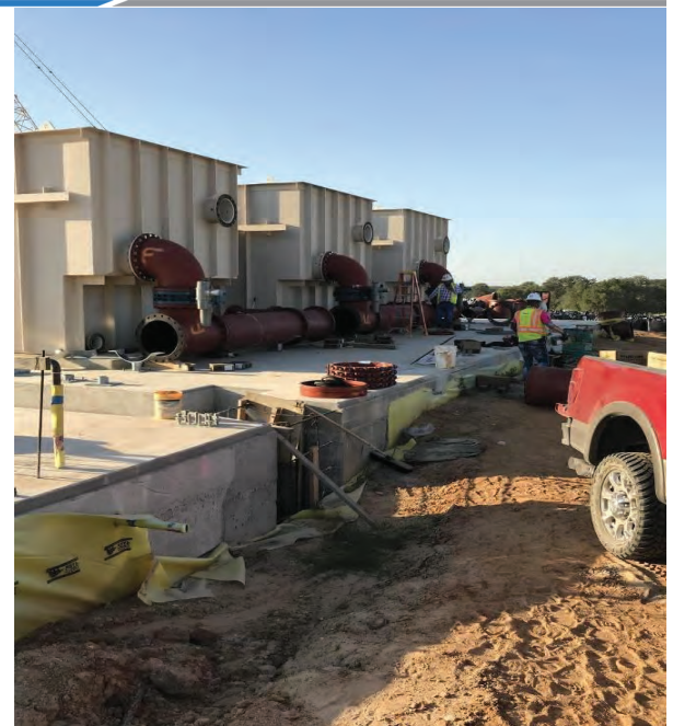
WTP - Filter Unit Process Piping
