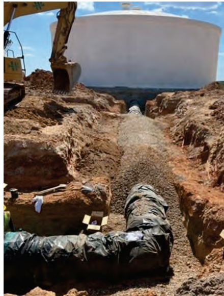
WTP – 36" Ground Water Piping to GBRA Raw Water Tank, Backfill with Gravel.
