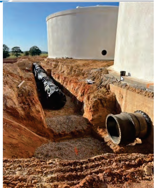
WTP - 36" from Tee Toward ARWA Tank
