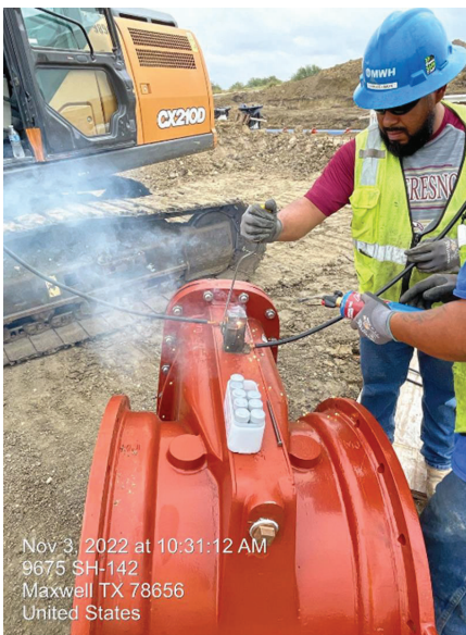
BPS – Cathodic Protection for Seg D 24" Gate Valve STA 12+86
