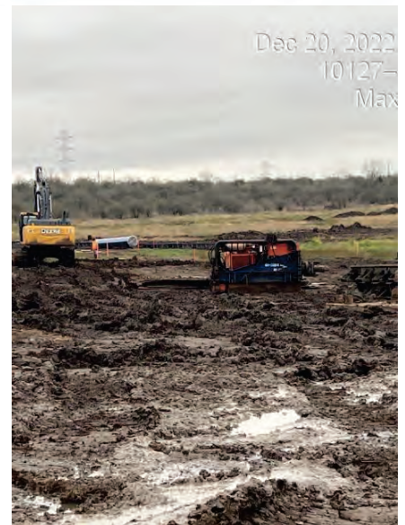
Seg D – Equipment Set Up
