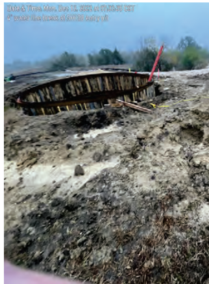
Seg B – SH130 – 4" Water Line Break at Entry Pit
