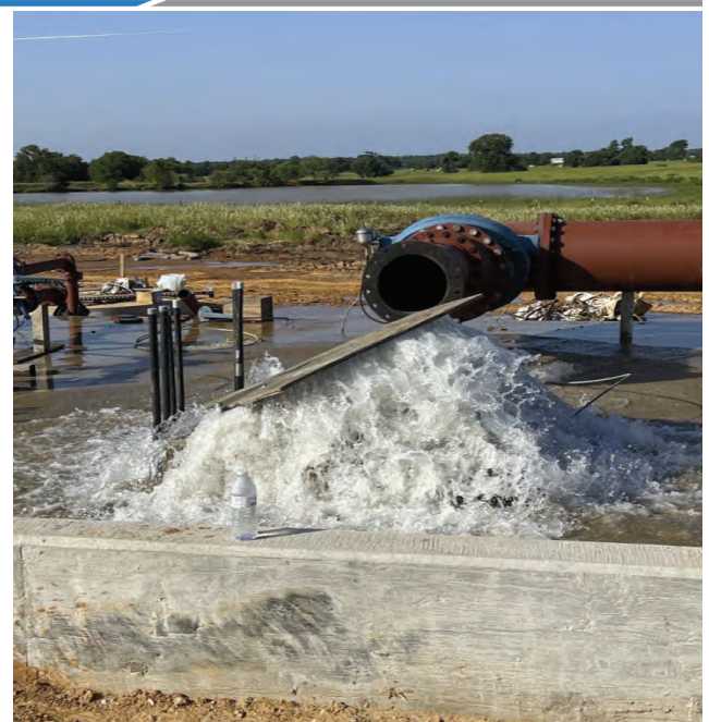
WTP - HSPS Flushing Pump Cans
