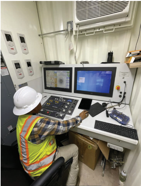
Seg A – Melcar’s Conducts Communications Check in Control Room
