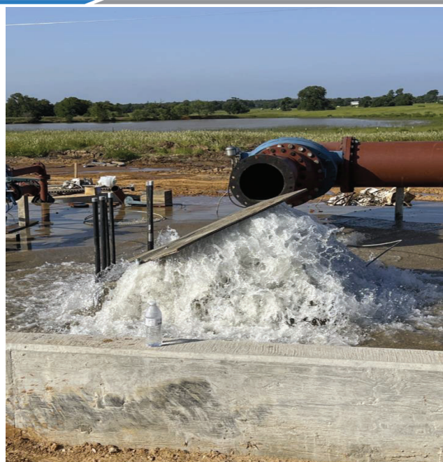
WTP - HSPS Flushing Pump Cans
