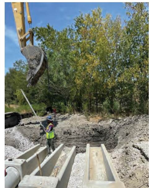
BPS – Detention Pond Outfall
