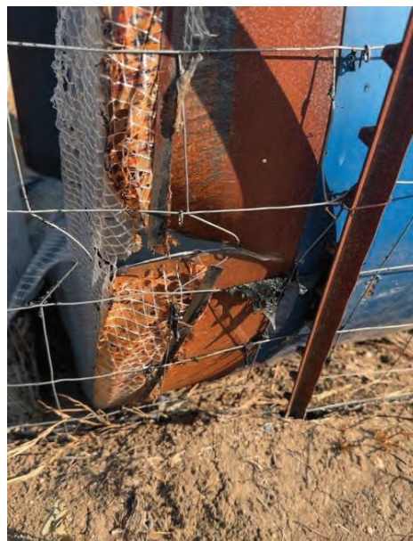
Seg B – Pipe Damage from Fire
