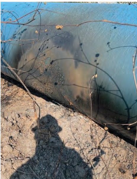
Seg B – Pipe Damage from Fire
