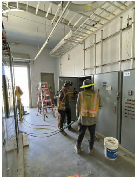
BPS - Wire Pull for Pump Soft Starts
