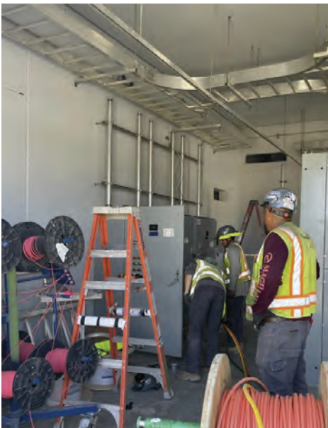
BPS – Wire Pull for Pump Soft Starts
