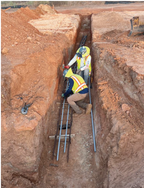
WTP – Installing Conduits for Lighting Duct Bank South Side of Lime System
