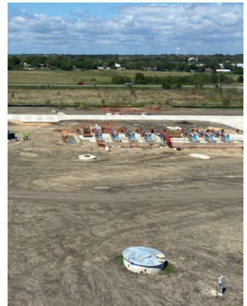
BPS – Booster Site from Ground Storage Tank 8
