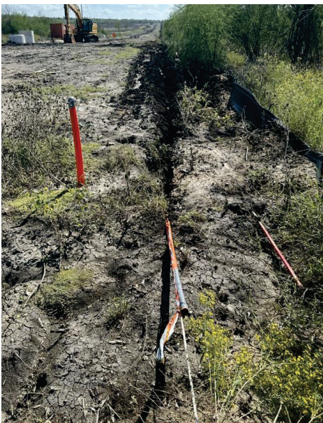
Seg B – Start of Fiber Optic Duct
