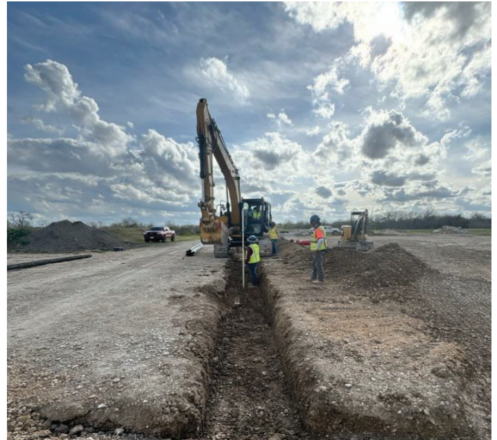
BPS – Chlorine Analyzer Drain Line
