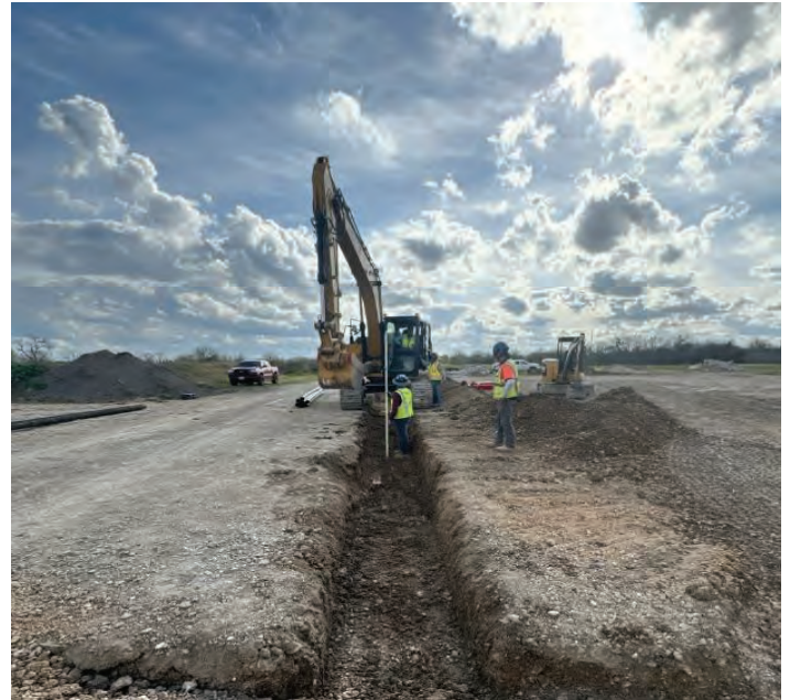
BPS – Chlorine Analyzer Drain Line
