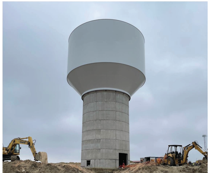
EST – Elevated Tank in Resting Place
