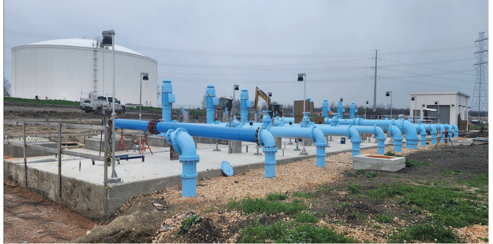
BPS – Pump Station Piping
